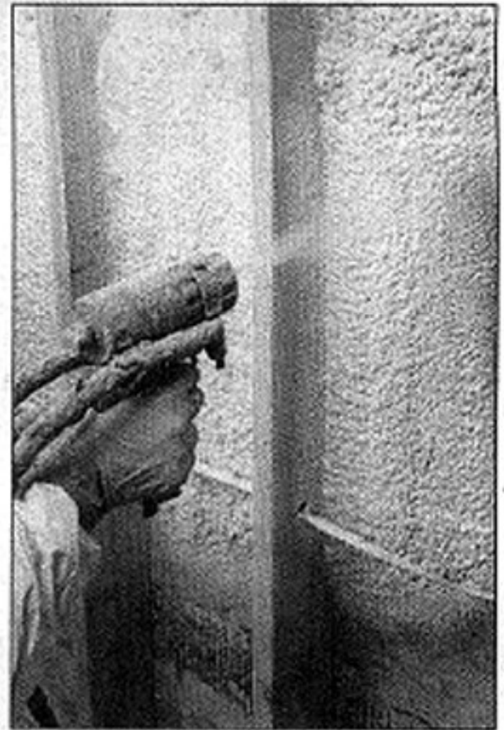
David W. Harple/Staff photographer Foam insulation is sprayed onto the interior walls of a new house in New Milford on Tuesday.
